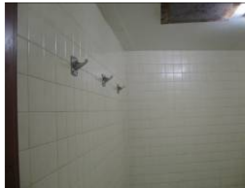
Unsafe Rigid Shower Hooks
