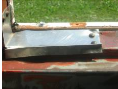
“Repaired” Metal Window Frame
