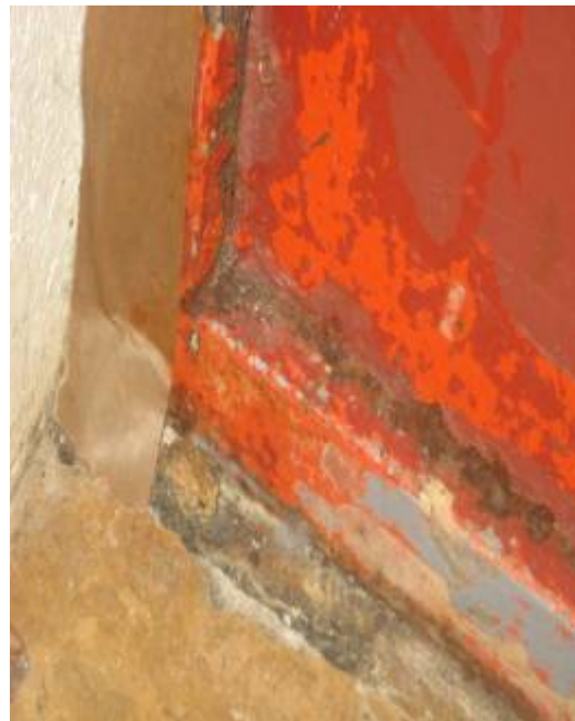
Close-up of Metal Plate
