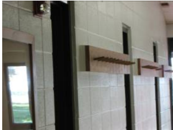
Unsafe Coat Hooks in Dayroom
