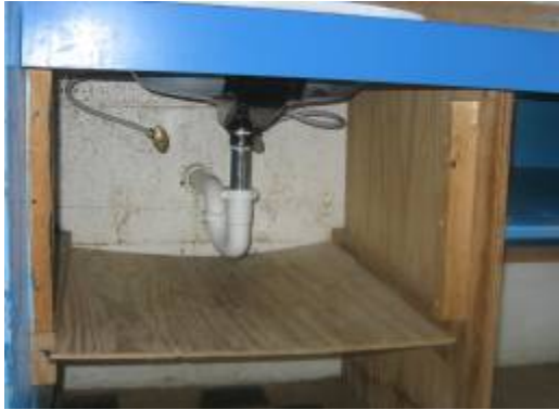
Exposed Unsafe Sink Pipes
