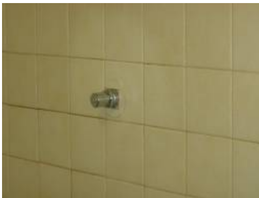
Unsafe Shower Control
