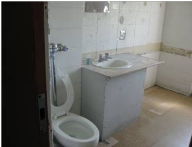
Unsafe Porcelain Toilet and Sink
